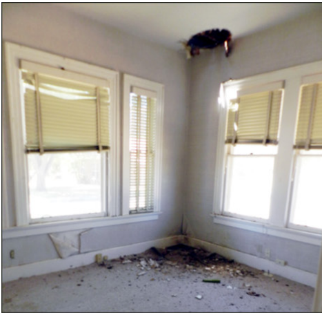
Interior damage of Kerrville Medical Center.
